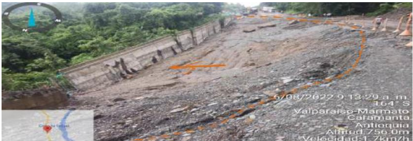
Figure 1. Damage and failure of the containment structure as of Aug 6, 2022
